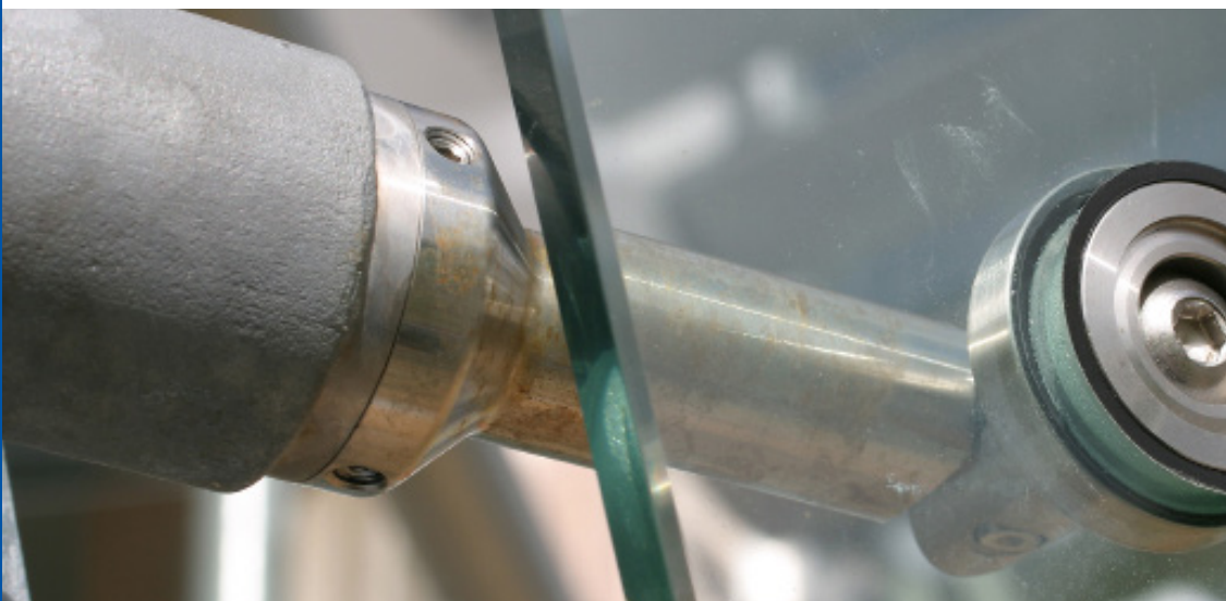
Stainless steel in direct electrical contact with galvanized steel which may result in bimetallic corrosion
